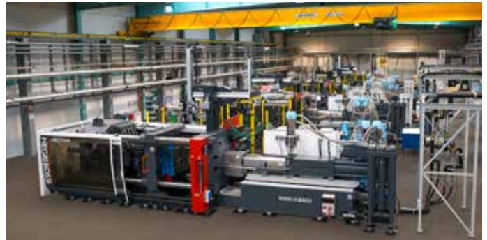
Injection-moulding plant II
